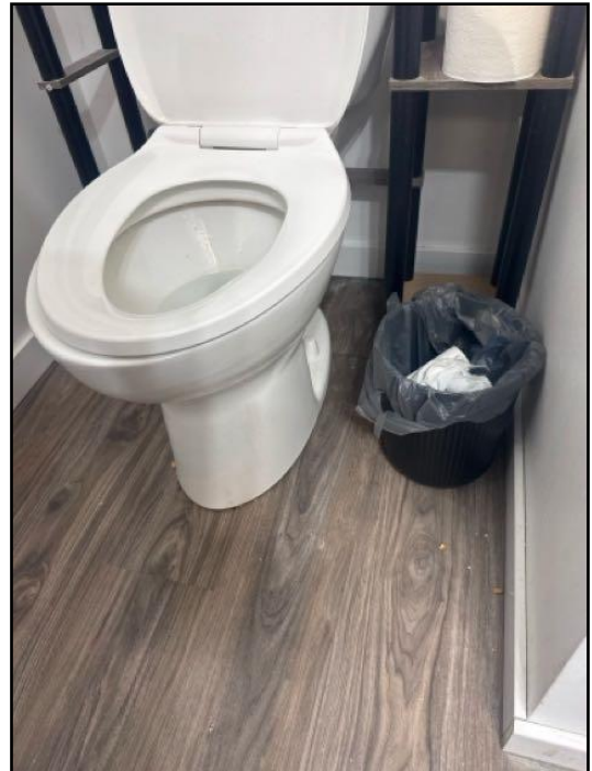
77. Floor damage suspected
