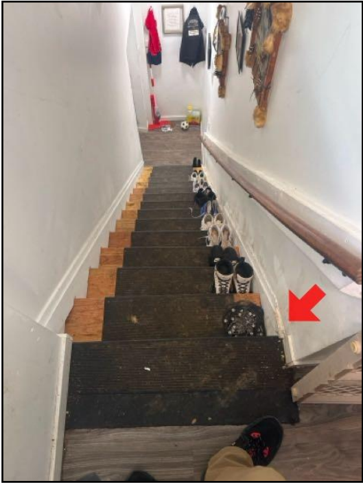
89. The building shows sign of structural...
