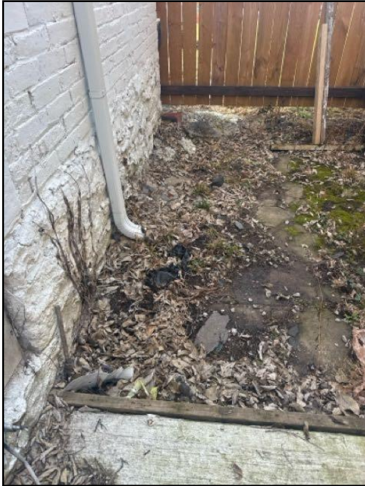
28. Improper slope or drainage
