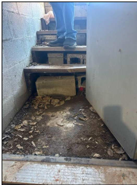
27. The basement stairs are not uniform, with...
