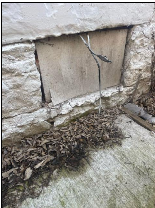
18. The windows are sealed shut. This lack of...
