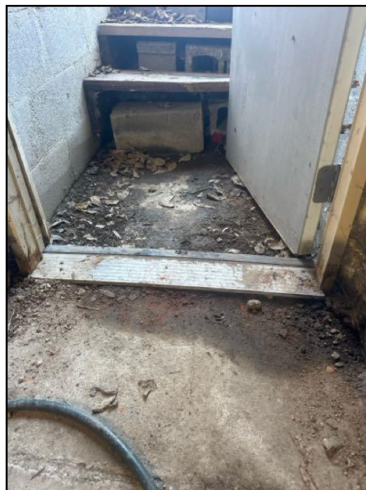
26. Door threshold missing, too low, not...
