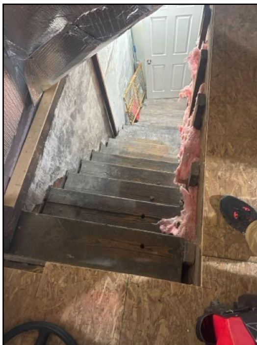
90. Worn or damaged
