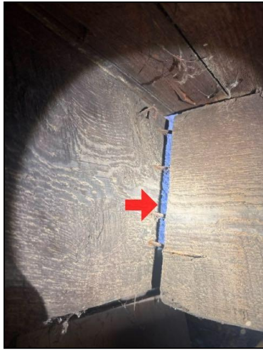
35. Poor end bearing, joist hanger connections
