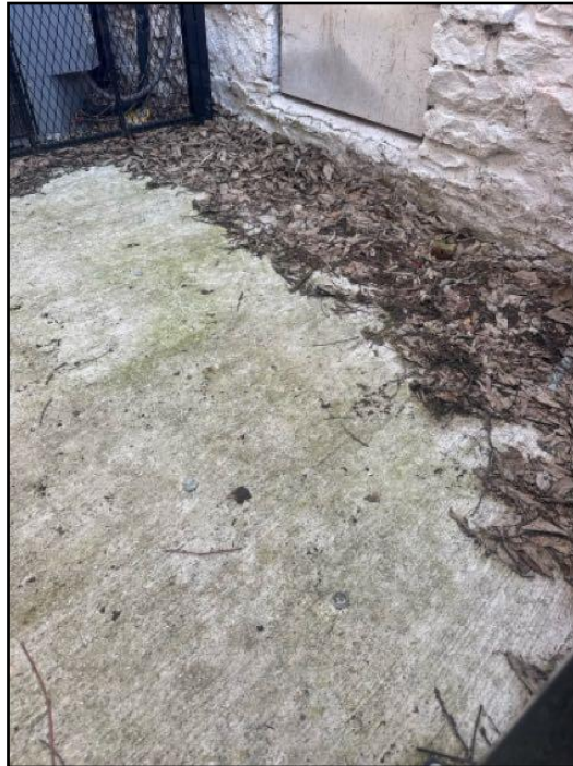
30. Improper slope or drainage
