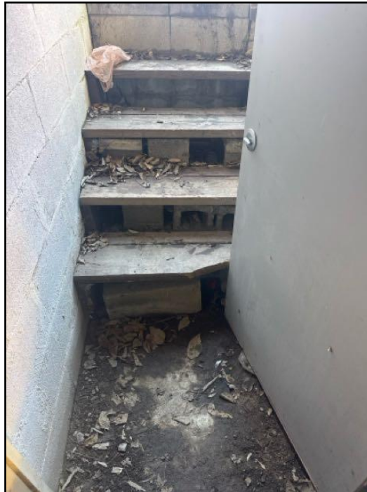
25. The basement stairs are not uniform, with...
