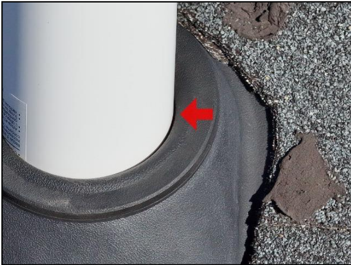
8. The pipe boot collars exhibit signs of...
