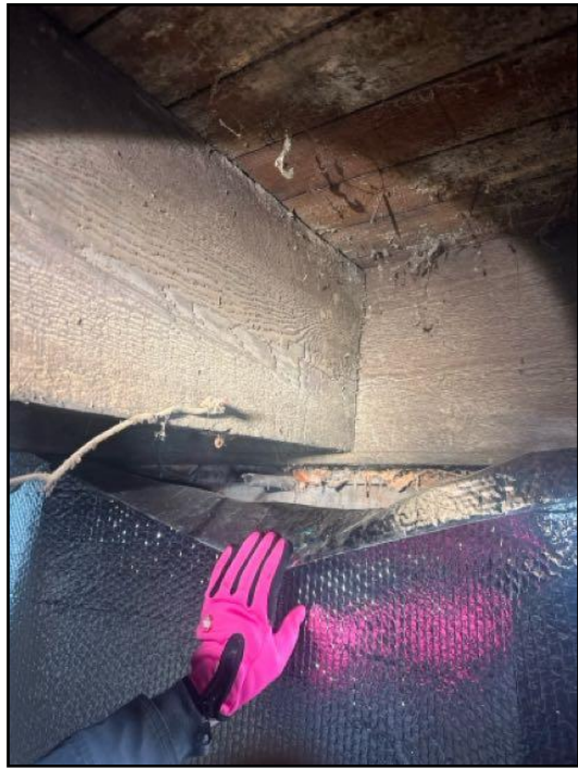
34. Poor end bearing, joist hanger connections
