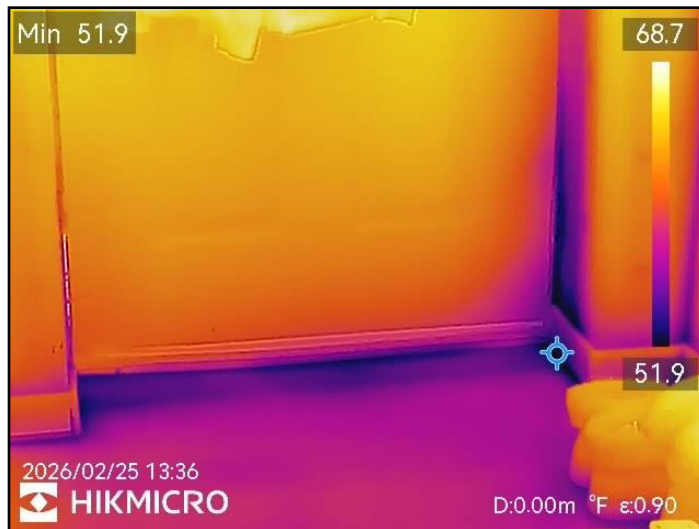
87. Weatherstripping missing or ineffective
