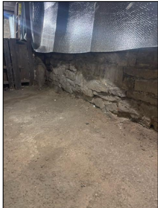
94. You need to be aware basements below grade...
