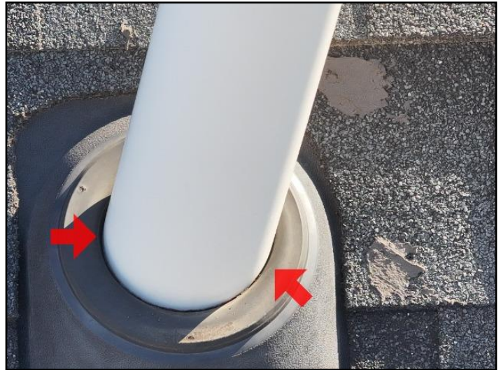
9. The pipe boot collars exhibit signs of...
