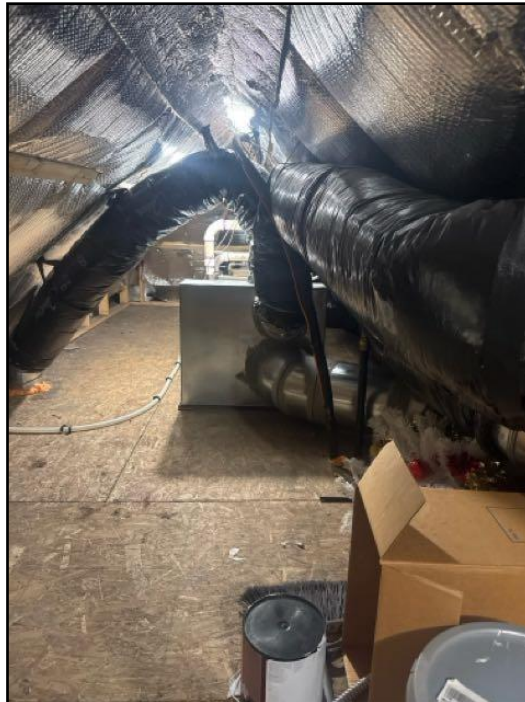
55. Attic service receptacle is not present. In...
