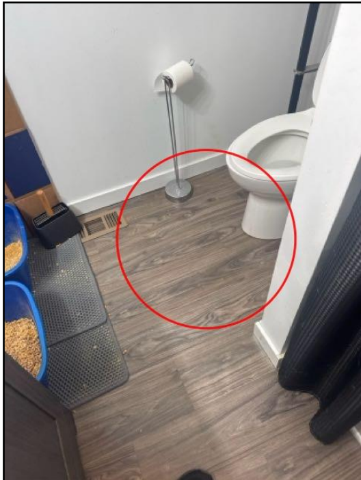
76. Floor damage suspected
