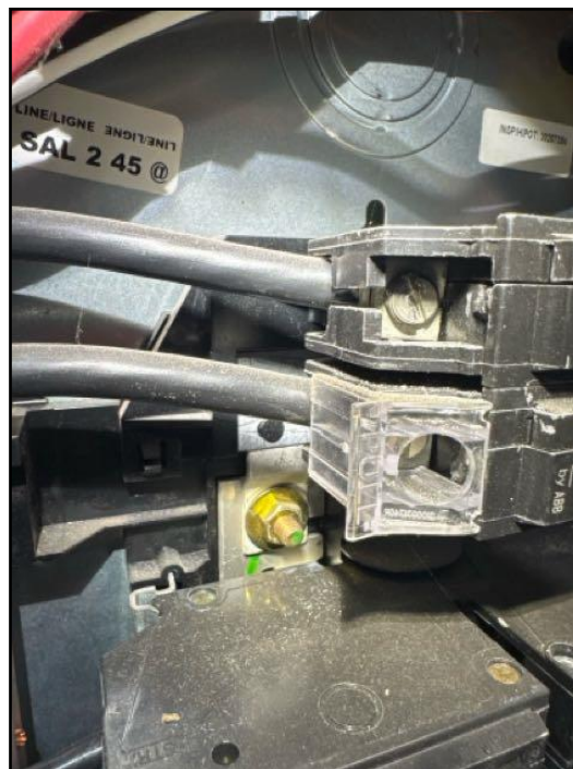
45. Anti-oxidant missing on aluminum wire
