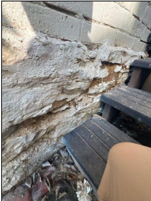
91. You need to be aware basements below grade...
