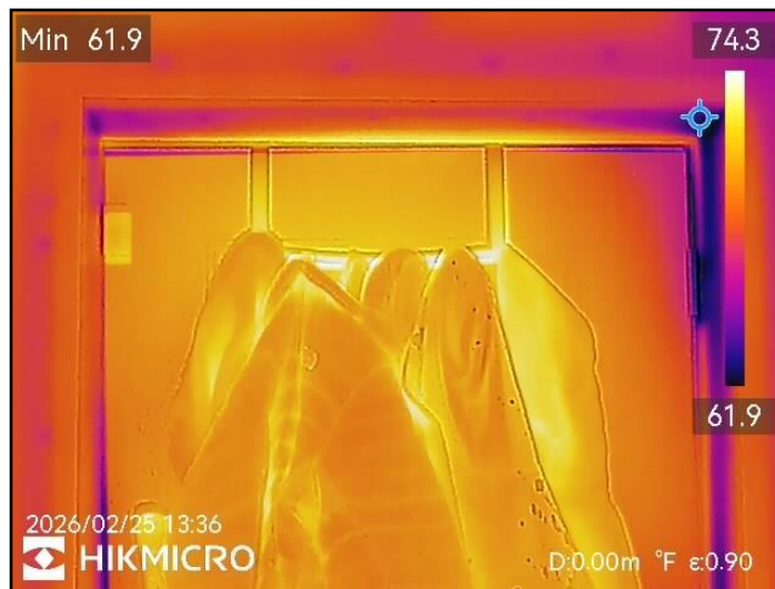
88. Weatherstripping missing or ineffective
