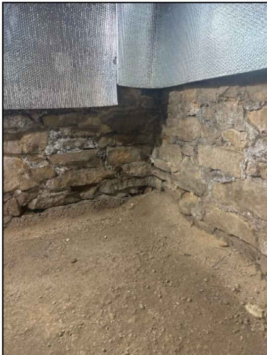
93. You need to be aware basements below grade...
