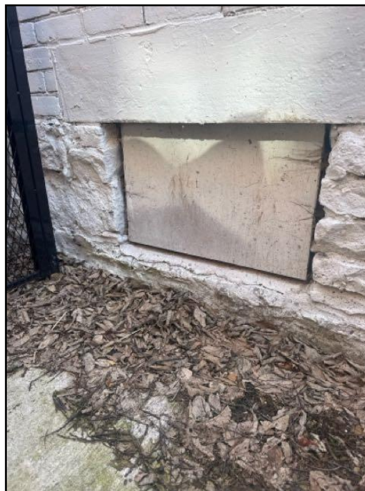
19. The windows are sealed shut. This lack of...
