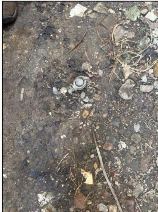
37. Copper - ground rods
