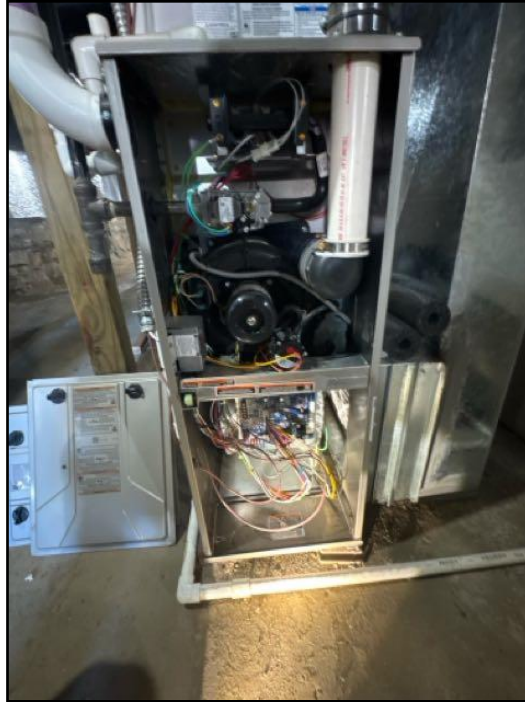
46. All readily openable access panels were...
