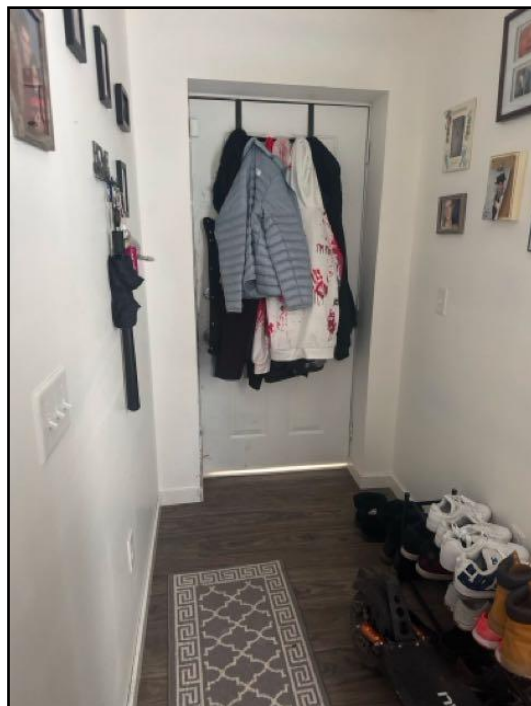
86. Weatherstripping missing or ineffective
