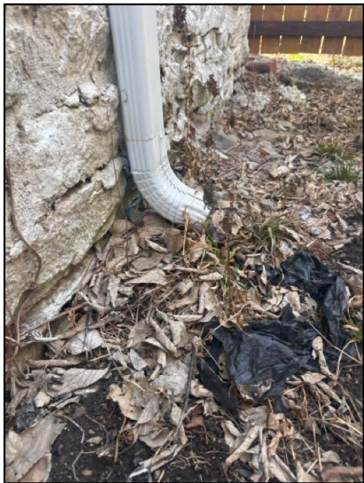
11. Should discharge 6 feet from building
