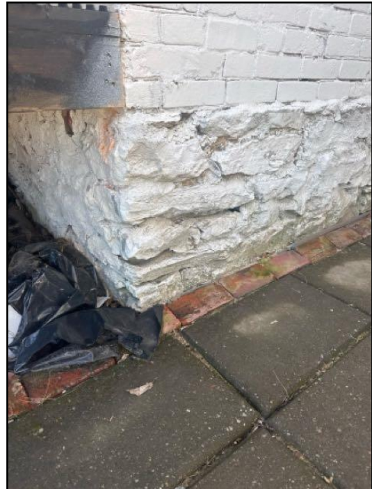
92. You need to be aware basements below grade...
